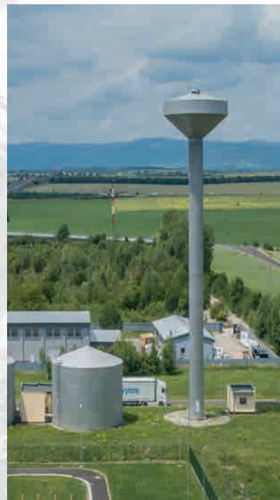
The water tower with drinking water and the water tank of treatment water / vodojem s pitnou vodou a zásobník průmyslové vody
